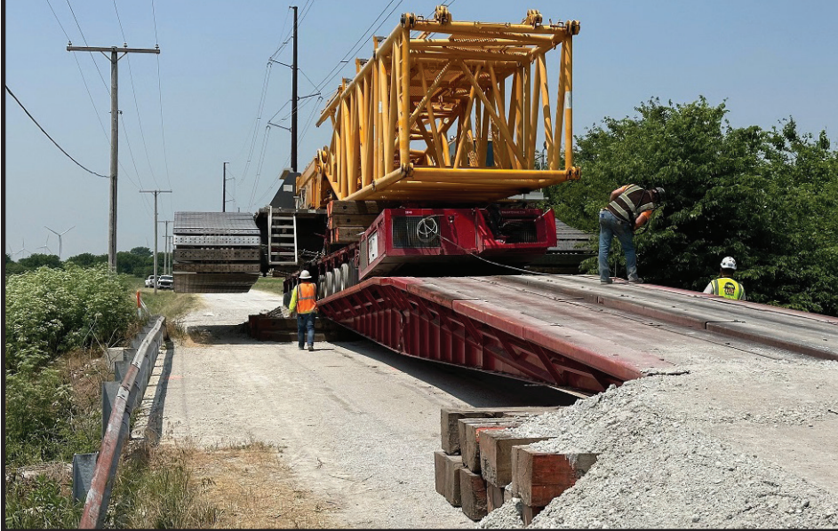
Local 103 Operators moving a LR1600-2 across a county bridge with 536,000 lbs on the SPMT trailer.
